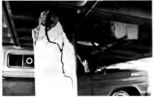
Photo 42. Carport collapsed on several ambulances.
